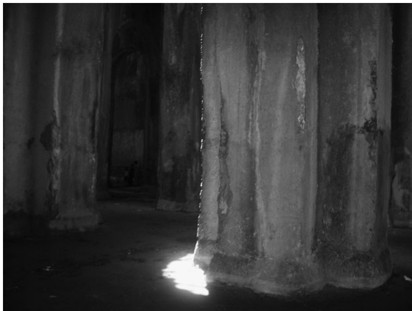
Fig. 6.2. Underneath Bacoli: the so-called Piscina Mirabile ('marvellous pool'), a system of subterranean Roman cisterns (photo: Giovanni Lombardi).
