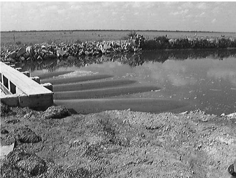
Fig. 15.10. Screens are used on both intake and discharge canals.
